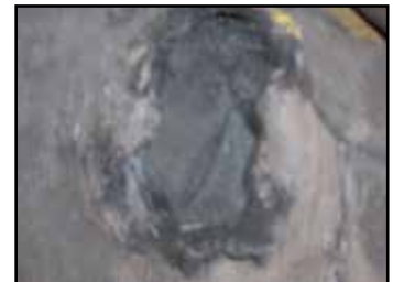
Melted or Charred areas
